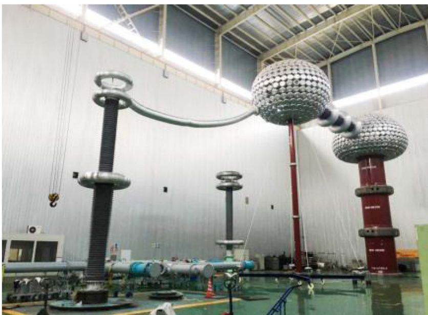
1650kV Power frequency system
