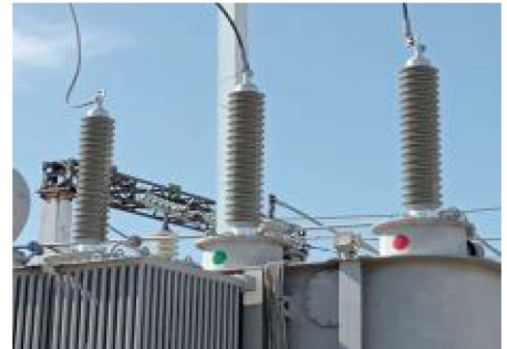
145kV RIP Bushings
