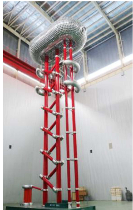
±2400kV DC system
