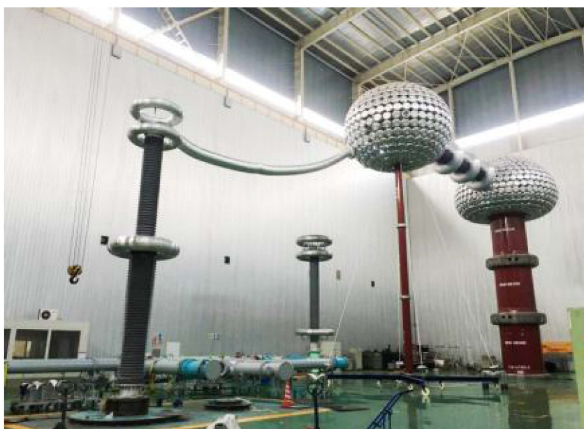
1650kV Power frequency system
