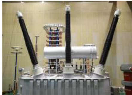
550kV OIP Bushings
