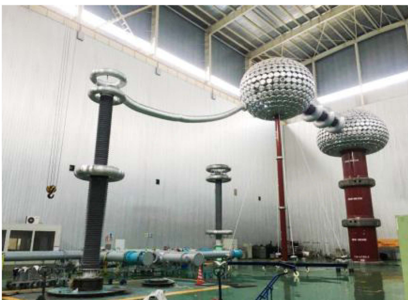
1650kV Power frequency system
