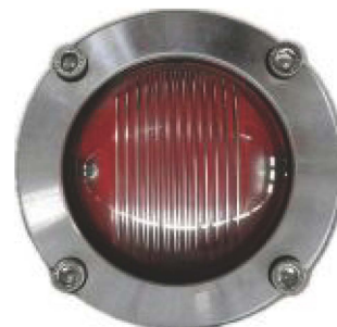
Oil level too low
