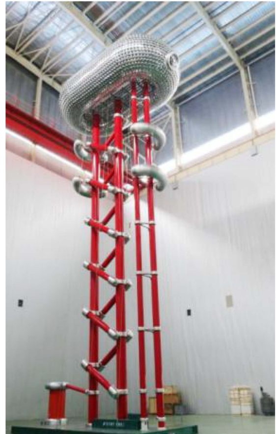
±2400kV DC system
