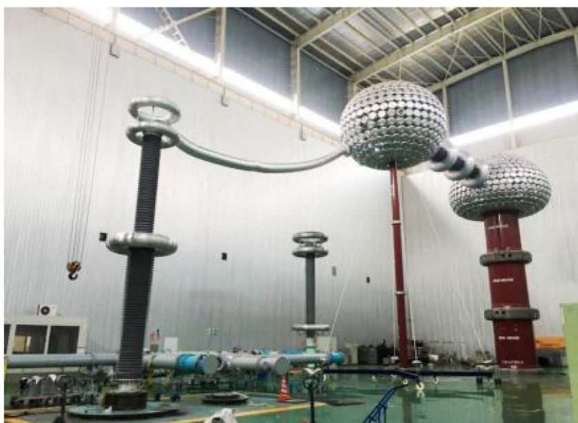
1650kV Power frequency system
