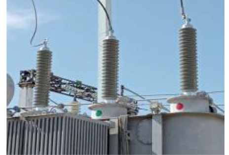
145kV RIP Bushings
